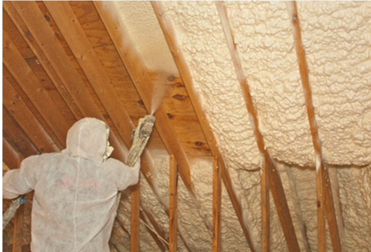
Figure 2. Application of Enverge EasySeal Ultra Spray Foam Insulation in an Unvented Attic
